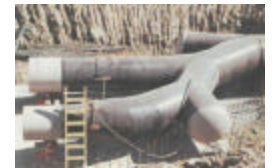
Pipelines as both municipal and irrigation water supply systems
